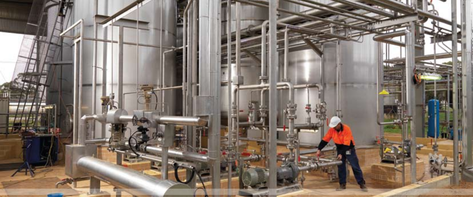
Mixed Acid Process Plant, New South Wales
